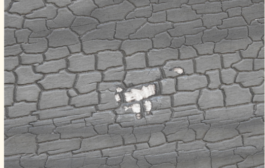
Close-up of damaged SSB Gator®
