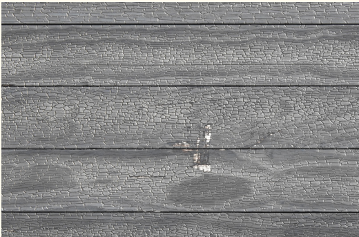
Damage from a ladder - scraped SSB Gator®
